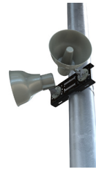
Dual Paging Horn installation
